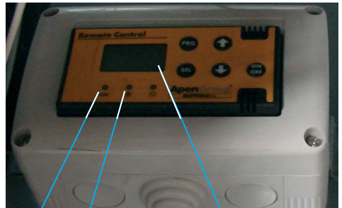
Unit switched on Gas in operation Instantaneous voltage display screen
