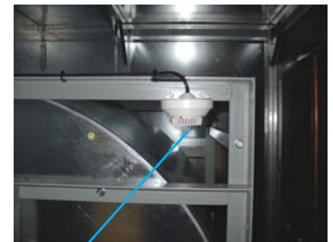
Smoke detecting station
