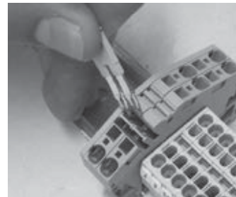
Removal of shunt to deactivate a heater (drop of 1000W)
