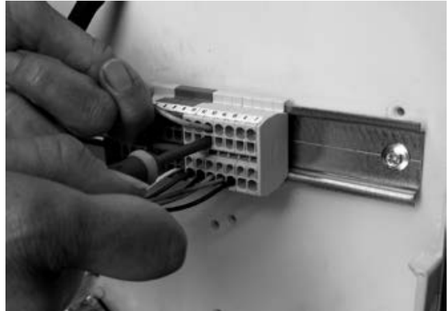
The customer must cable the speeds for the thermostat at the top of the terminal block between V1 and V5
